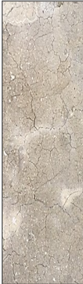
Fig. 3 Cracking After Subjecting to High Temperatures.
