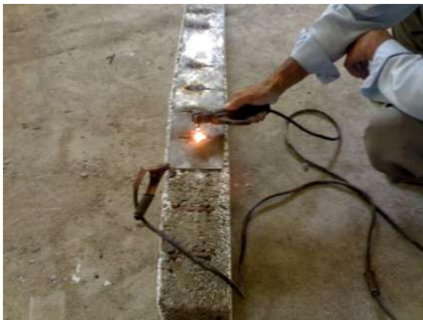
Figure.(4) Welding the steel plate to the stirrups at the tension face
