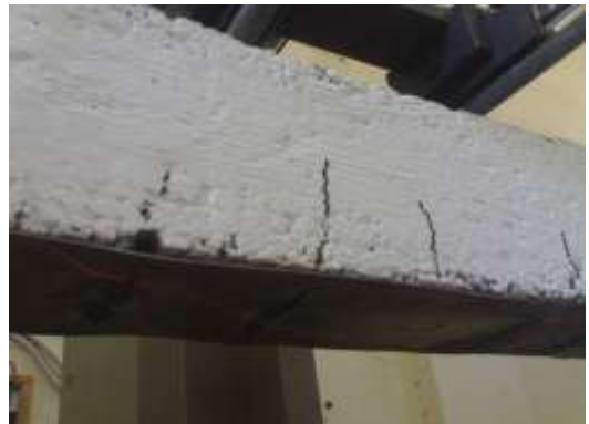
Figure. (14) View of Cracking of Beam B10 (100%Preloading, debonding in one welding point)
